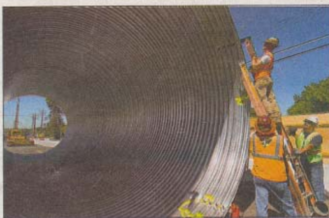
Workers prepare to raise a 55-foot-long section of pipe that will be lowered into a shaft in Citrus Heights. The hole was drilled by an enormous auger nicknamed "Big Stan," which can be seen in the background on the left.
