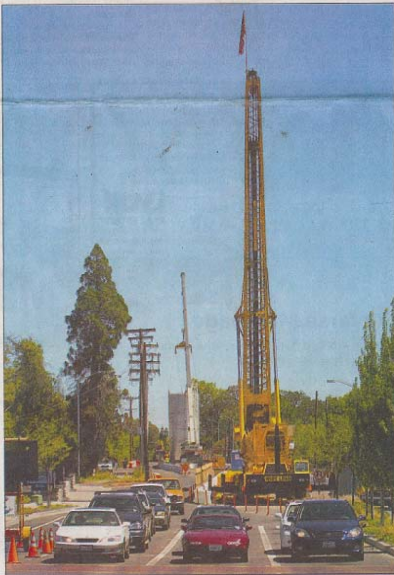
A 93-foot auger known as "Big Stan" is being used to drill shafts for a sewer project in Citrus Heights. The drill, featured on TV, can create holes up to 30 feet in diameter.
